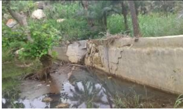
Kozha (Kara) Dam poorly designed, to be taken over by NGO
